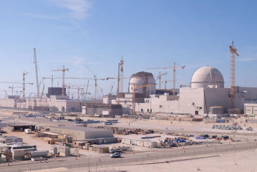
Construction of UAE's first nuclear power plant at the Barakah site. L. POTTERTON / IAEA.
